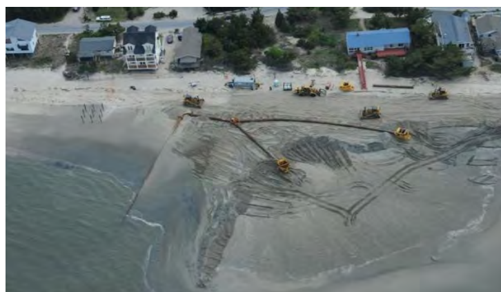
An aerial view of the USACE beach renourishment project at Broadkill Beach
