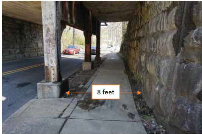
Figure 10: Existing sidewalk under railroad bridge along West 18 th Street, looking south/east; clearance between pier and wall measures 8 feet.
