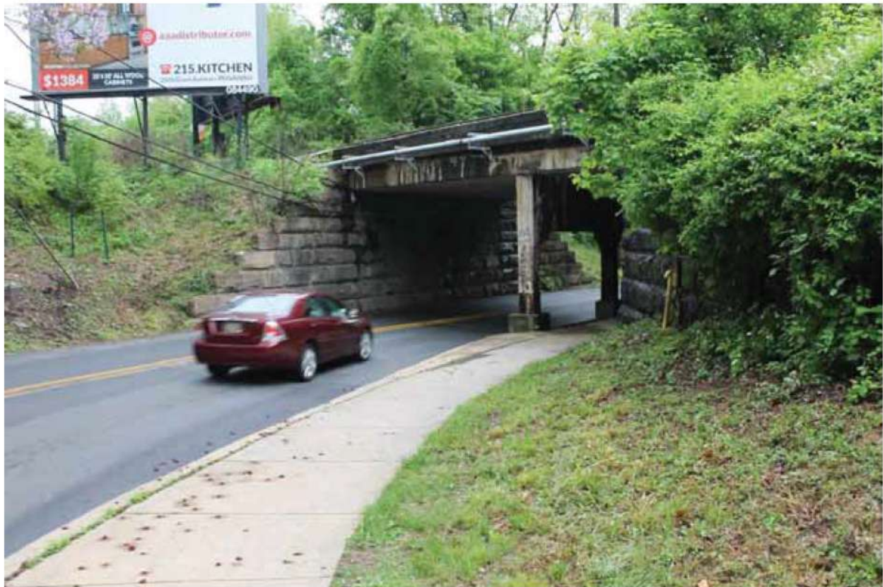
Figure 11: Approach to the railroad bridge underpass on West 18 th Street from the north side of the bridge. Limited sight lines and a narrow passage should be addressed by alerting users with pavement markings, signage, and other methods.
