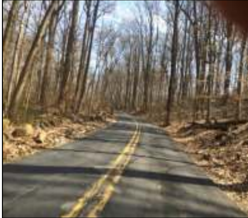
This picture of Ramsey Road shows the narrow travel lanes and the drainage ditch along the roadway on the right side of the picture. Also shown is the proximity of the large boulders on the left side. This section of Ramsey Road is in the First State National Historical Park.
