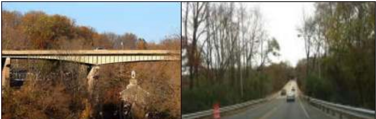
Views of the Tyler McConnell Bridge that carries DE Route 141 across the Brandywine Creek. The structure has been deemed historic to the National Register of Historic Places. This presents challenges in either a replacement or in offering a twin structure that may or may not be harmonious to the viewshed and of other historic properties as seen from below.
