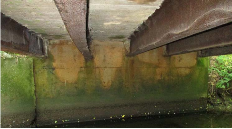
Photo 20: View of existing bridge beams with impact and horizontal translation of the lower portions of the beams
