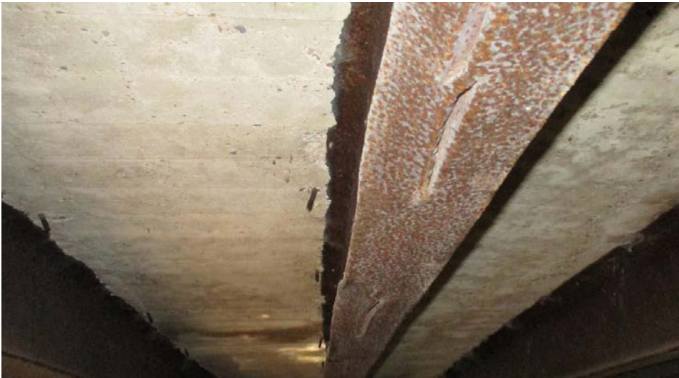
Photo 21: View of existing bridge beams with longitudinal tears
