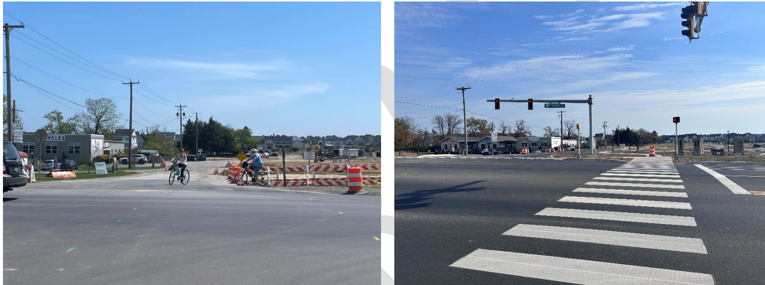
Figure 12. The intersection of Freeman Highway and Monroe Avenue during and after developer intersection improvements were installed
