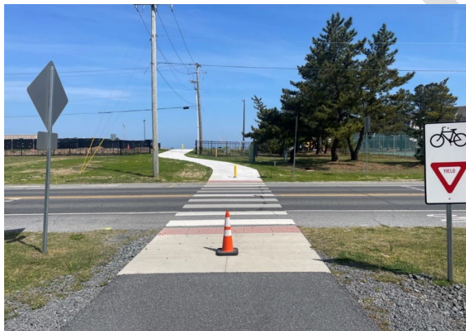
Figure 7. Newly installed crossing connecting the Lewes Ferry Terminal with the Georgetown–Lewes Trail across Cape Henlopen Drive
